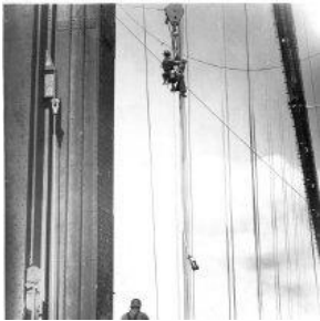
Object Name: Print, Photographic Date: 1940 Description: Bridge construction; worker climbing wires; man on deck Photographer: Bashford, James Copyright: Photograph by James Bashford Collection: James Bashford Collection Search Terms: Galloping Gertie Collection; Narrows Bridge - 1st bridge; Narrows
