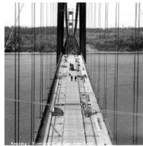
Object Name: Print, Photographic Date: 1940 Description: Roadway form work on east side span. Photographer: Bashford, James Copyright: Photograph by James Bashford Collection: James Bashford Collection Search Terms: Narrows Bridge; Gig Harbor; Galloping Gertie; Galloping Gertie
