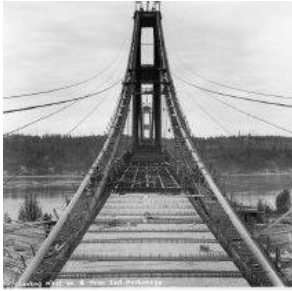
Object Name: Print, Photographic Description: First Narrows Bridge (Also known as Galloping Gertie) under construction looking west, toward Gig Harbor, while on and from east anchorage. Photographer: Bashford, James Print size: 8" x 10" Copyright: Photograph by James Bashford Collection: James Bashford Collection
